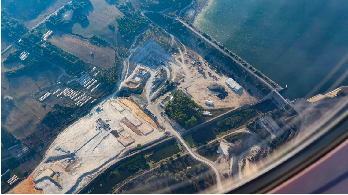
Photo 1. Sazlıdere Damlake, the construction site and sazlıdere stream from airplane on 16 Aug 2021. 10 species of birds were observed flying from north (right upper corner) to south (left lower corner) on daily basis.
